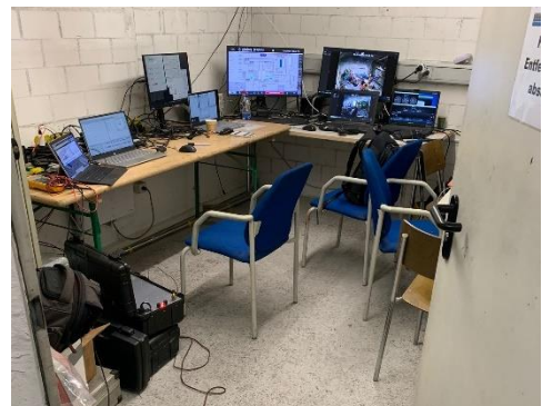
Fig. 12: Control room for data acquisition
